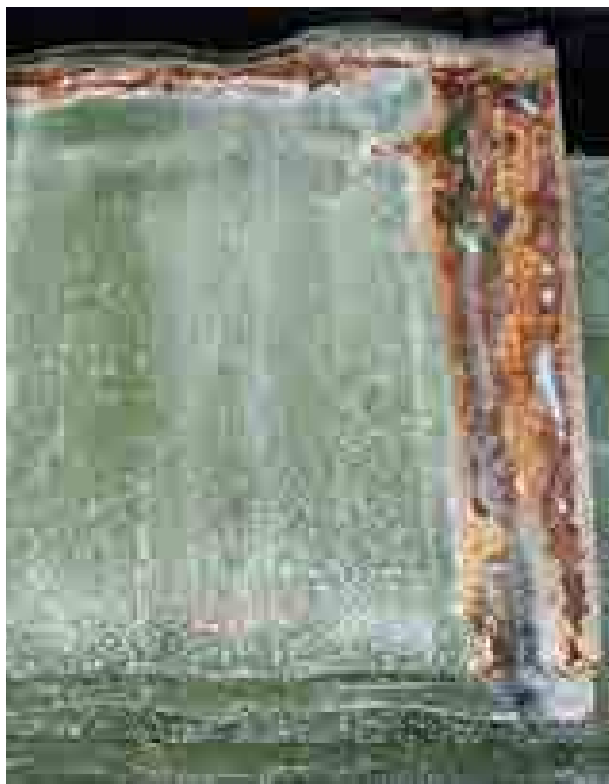
THIS PANEL SHOWS WHERE THE ZINC HAS ERODED AWAY AND THE RED RUST HAS TAKEN HOLD.
