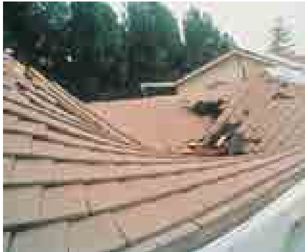
IN LOS ANGELES, THESE CEMENT SHAKES SLIPPED CAUSING SIGNIFICANT STRUCTURAL DAMAGE.
